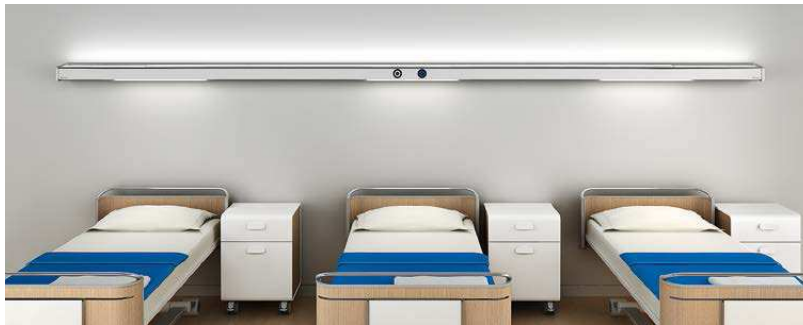
Caption 3: Three-bed room with continuous-row LED system (room light) and LED lighting modules (reading light/examination lighting).
